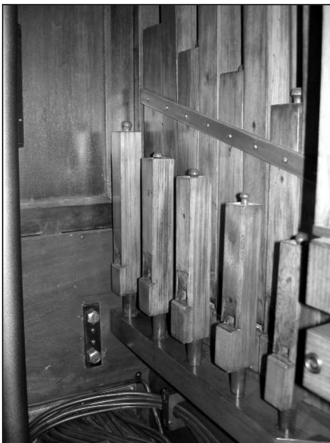
Figure 33. The back left group of accompaniment pipes. Just below is the inside keyframe tubing junction manifold.
