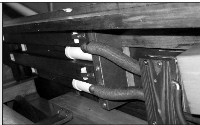
Figure 17. Two each of the replacement saxophone and cello helper pipes in their location under the roof of the case. Note the two supply conductors connecting the off-note chest fabricated for the operation of these two notes to the pipe table.
